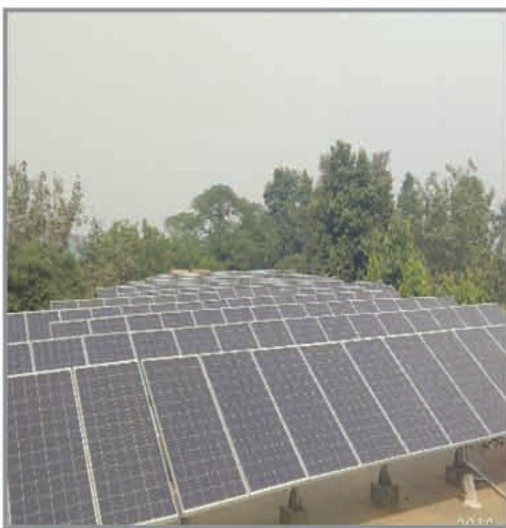
Solar Power plant is generating electricity for consumption of CTR
